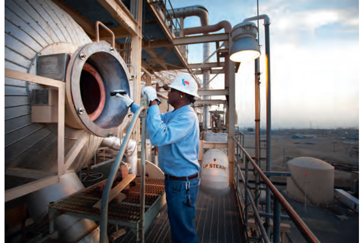
Engineer performing an inspection at CRC's power plant at Elk Hills Field near Bakersfield
