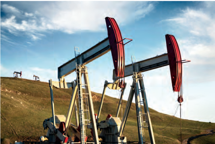
Pumping units at CRC's operations in Ventura
