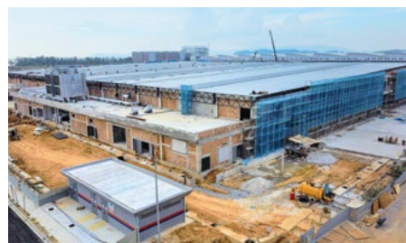
Work is progressing rapidly on our new high technology manufacturing facility in Penang, Malaysia.
