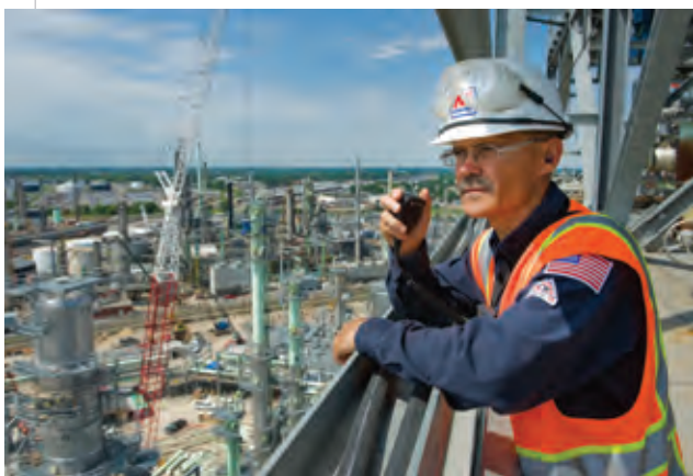
Advanced Senior Refining Engineer Pete Crews looks over the construction site at the Detroit Heavy Oil Upgrade Project from atop the refinery's new coker unit.
