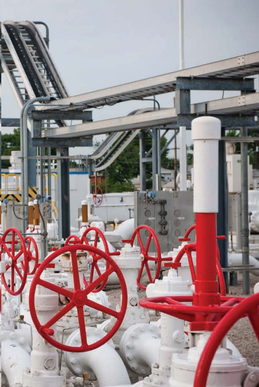
Pipes and valves at MPLX's Wood River, Ill., facility
