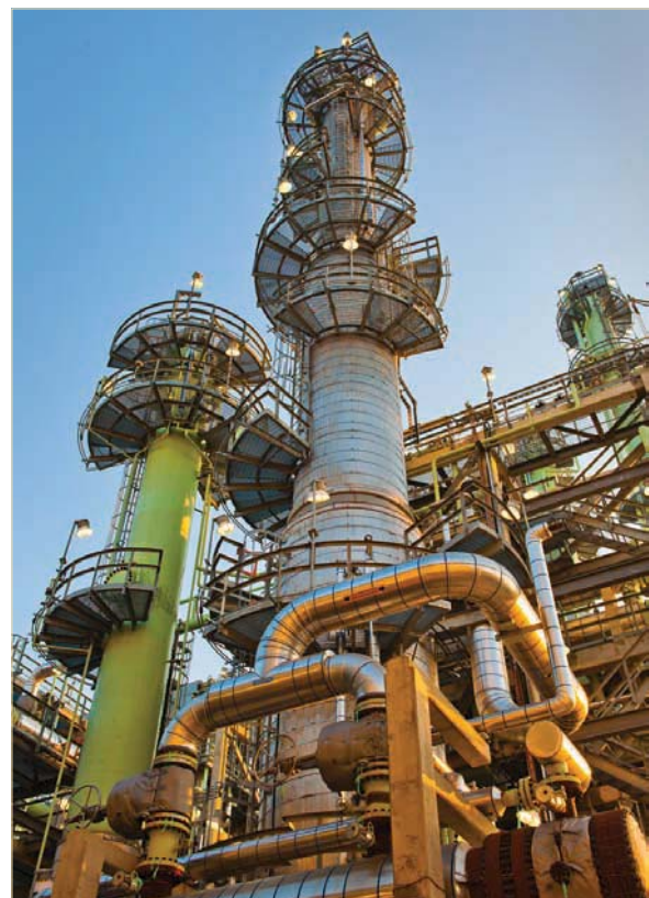
Right, new distillate hydrotreater at the Detroit refinery
