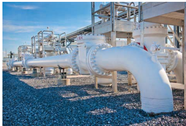
Left, pipeline at MPC's terminal near Garyville, La.
