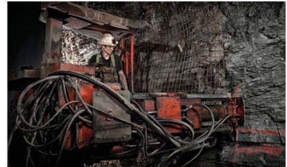
Above, construction on MPLX's 1 million bbl. butane cavern in Neal, W.Va., was completed in August.
