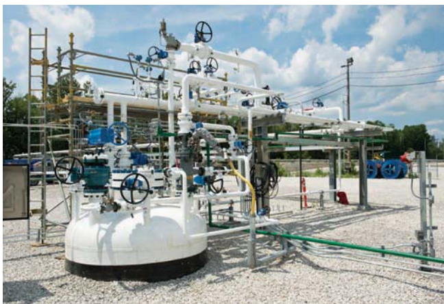
Above, main shaft double dome at MPLX's 1 million bbl. butane cavern in Neal, W.Va.
