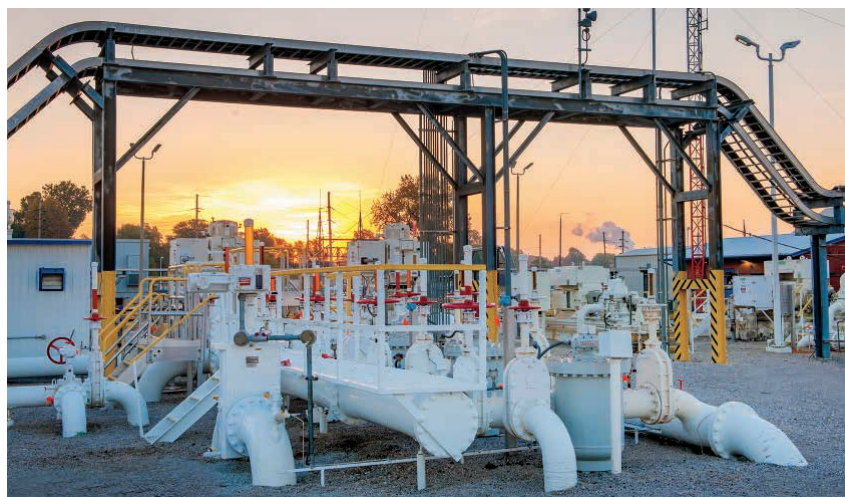
Pipeline infrastructure at an MPLX facility in Wood River, Ill.
