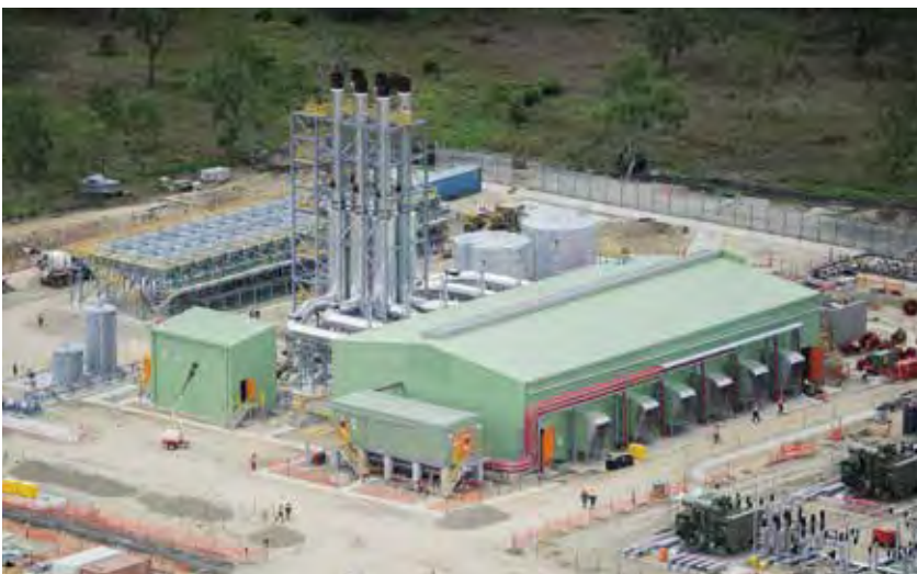
58 MW gas fired power station expected to supply approximately 75% of Port Moresby’s electricity needs.
