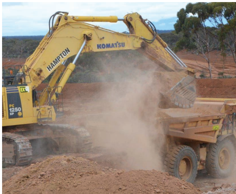
Photo 4: First stage excavation at the Cannon Gold Mine with 120 tonne Komatsu PC1250 Excavator loading a Caterpillar 777F 100 tonne truck.
