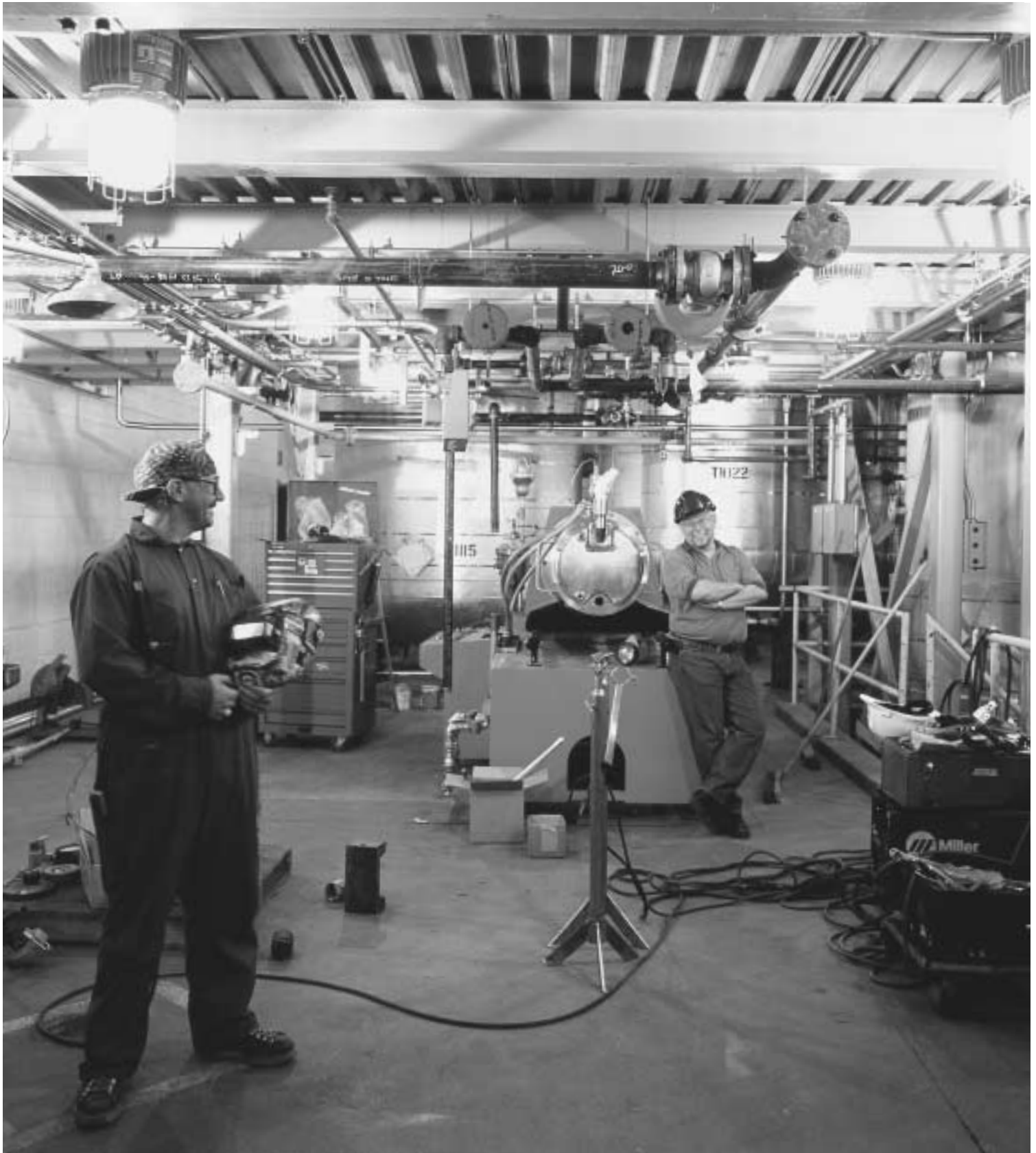
ABOVE: DENNIS PERRY, TRIANGLE STAINLESS CONTRACT WELDER, ON CALGARY'S REACTOR TRAIN UPGRADE WITH NUFARM PLANT MANAGER, DALE WINTER.
