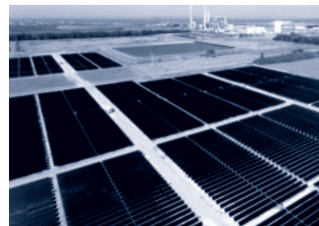
The 23 MW Big Bend Solar facility is the largest solar array in the Tampa Bay area.
