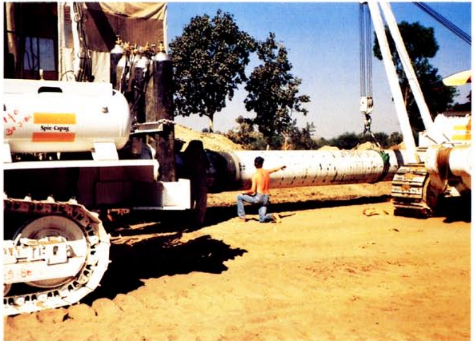
India: Work continues on the 1,700 kilometre HBJ gas pipeline project, for which the Group has won the banking business.
