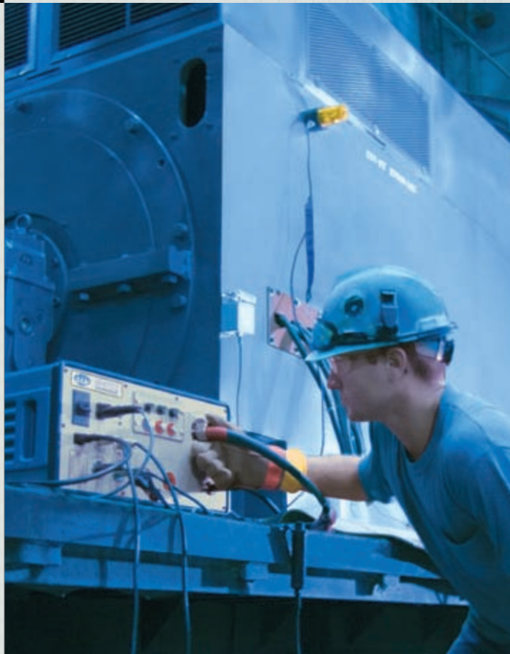
The "Doble Test" evaluates the condition of high voltage power apparatus as part of routine maintenance checks using the Doble M4000 analyzer.
