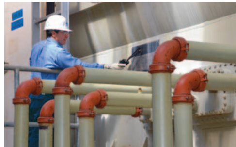
A Doble engineer performs on-site testing using Electromagnetic Interference Diagnostics™, an on-line survey that detects both electrical and mechanical defects in generators, motors, isolated phase bus ducts and transformers.
