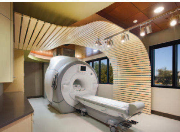
State-of-the-art MRI facilities require both high-quality shielding as well as first-class workmanship to meet the requirements of a demanding customer base.
