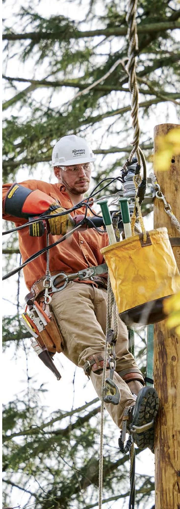
CEI line worker, Ben DeBottis, repairs windstorm damage in the Bay Village, Ohio, area.
