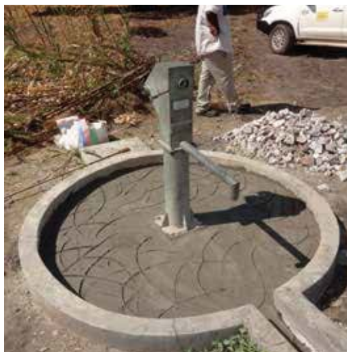
▲ Figure 9: Mechanical water boreholes
