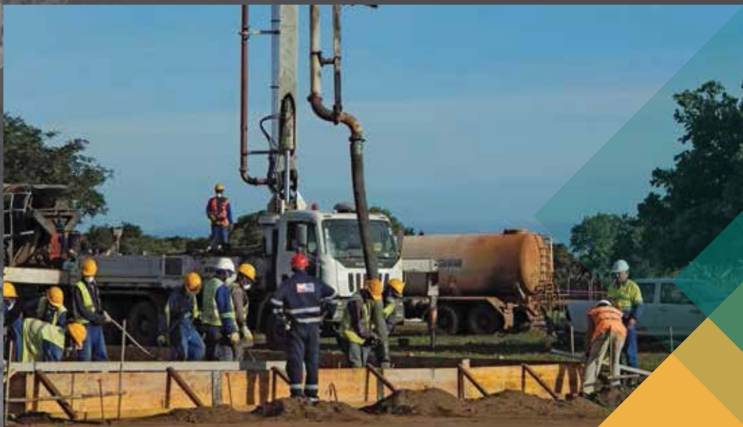
▼ Figure 4: Pouring of floor slab for the construction of a larger accommodation camp
