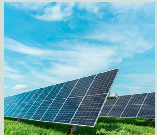
▲ Balama solar and battery project
