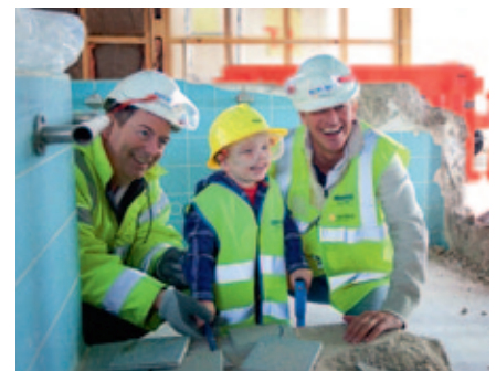
Ollie Saxton, a user of the Ryegate Children's Centre, assists Simon Carr, Henry Boot Construction, and Mark Dransfield, Dransfield Properties, in the demolition of the old hydrotherapy pool
