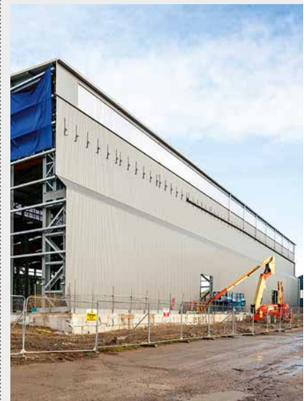
14,000m 2 of roof sheeting and wall cladding used to complete the press house
