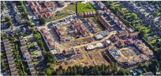
Ongoing development works at our successful site at St Albans in Hertfordshire
