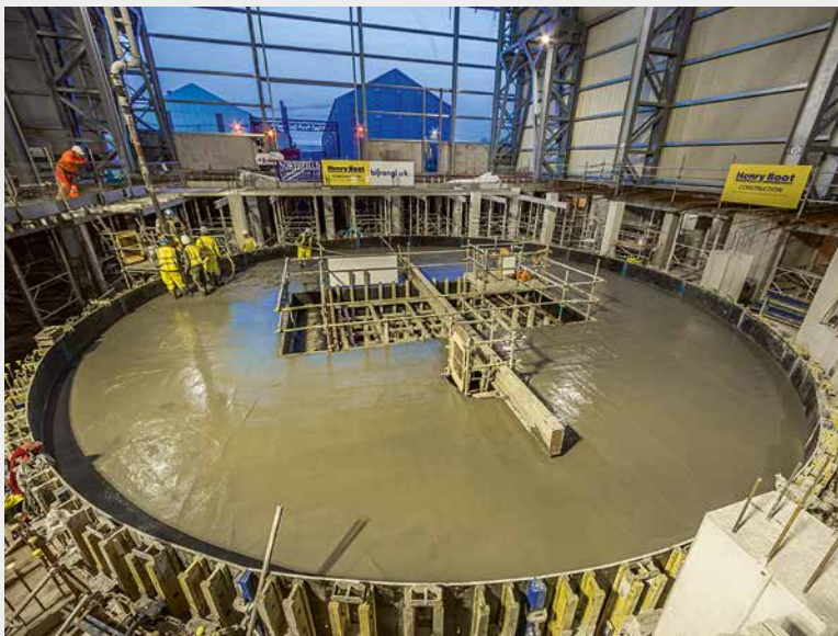
In February 2014 a 36 hour continuous concrete pour saw completion of the press block foundation
