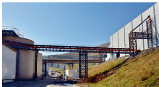
Tailings feed pipe from the agitation leaching plant (rear). The pipe to the main tailings disposal pipe is in the foreground.
