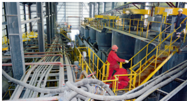
Inside of the flotation plant. The two conditioning tanks and six flotation cells are to the right and the 12 smaller flotation cells are to the left.
