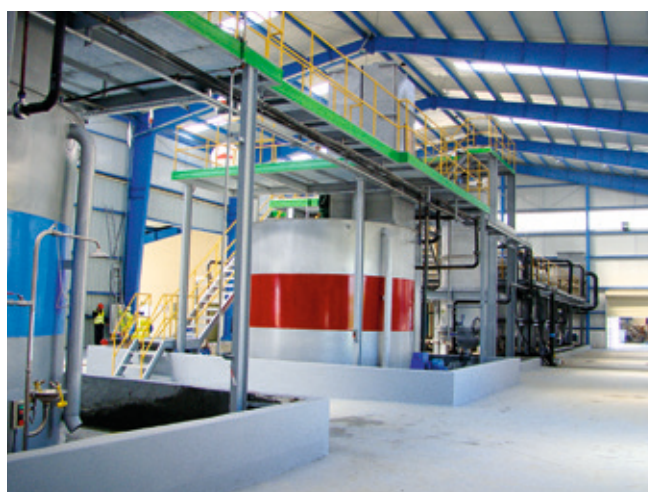
Inside of the SART plant.
