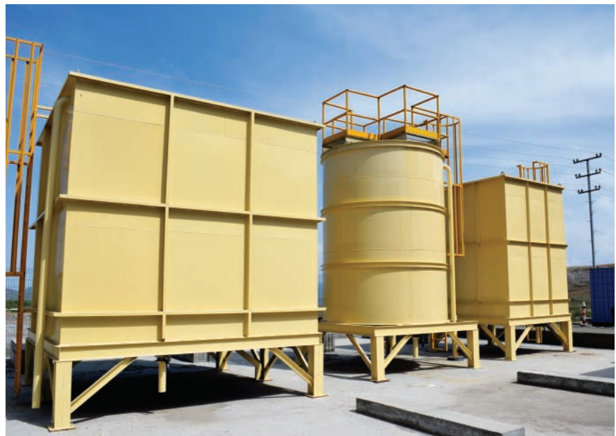
Newly installed tanks at the water treatment plant.
