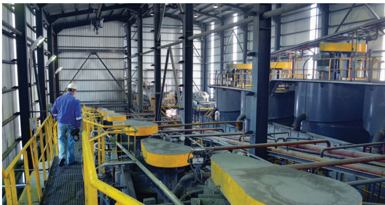
Inside view of the flotation plant showing the flotation cells to the right. The plant achieved its first full year of production in 2016.
