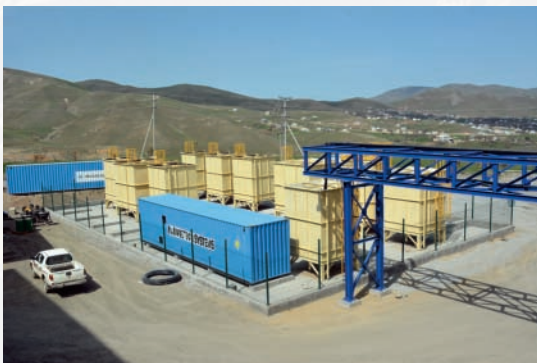
The new water treatment plant. The water filtration equipment is in the containers and the water tanks (yellow) can be seen. The gantry for the pipes between the water and processing plants can also be seen.
