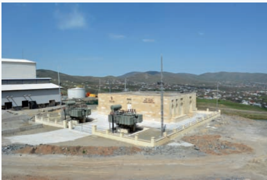
The new electrical power house and the two main electricity transformers.
