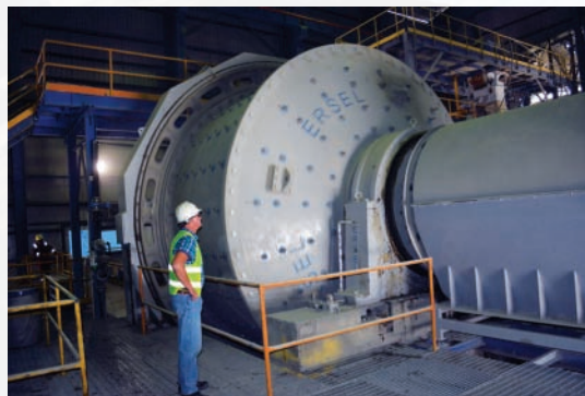
The second SAG mill in operation at the plant.
