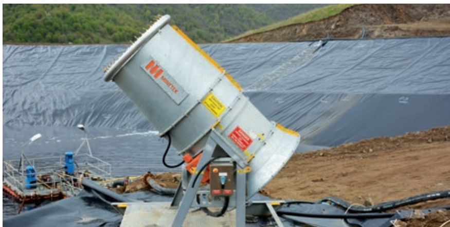
Waste water evaporator deployed in the tailings dam.
