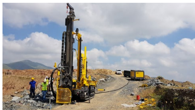
New drill rig deployed in the vicinity of the Gedabek open pit.
