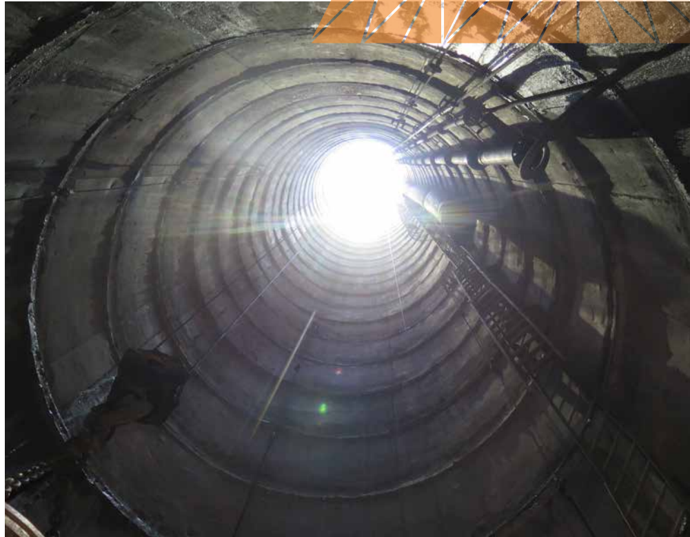
SPOTTED QUOLL PRIMARY VENTILATION RETURN AIR-WAY COMPLETION OF INITIAL 45M CONCRETE LINED SHAFT
