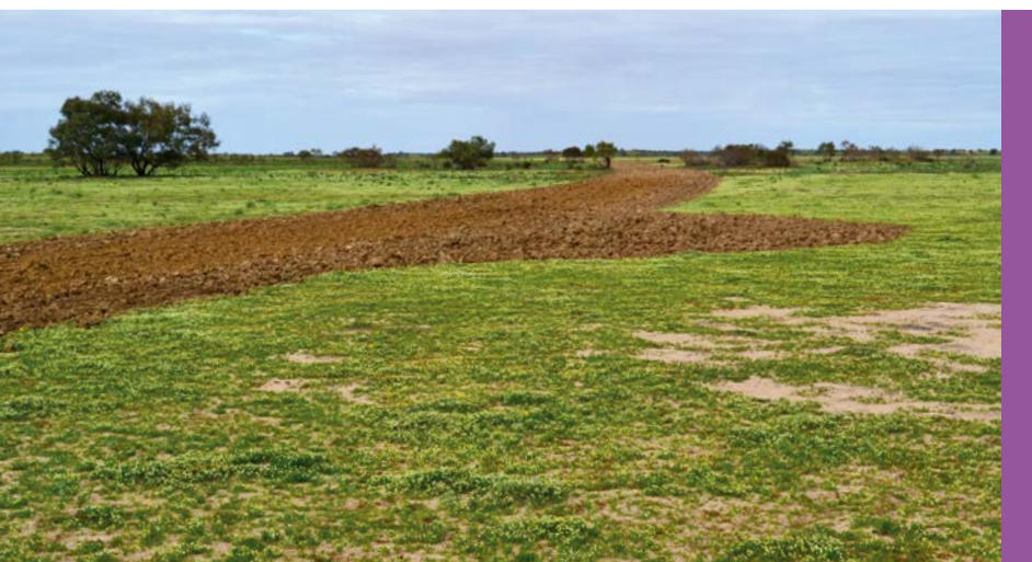
Rehabilitation earthworks with the edges being scalloped and blended into the surrounding landscape.
