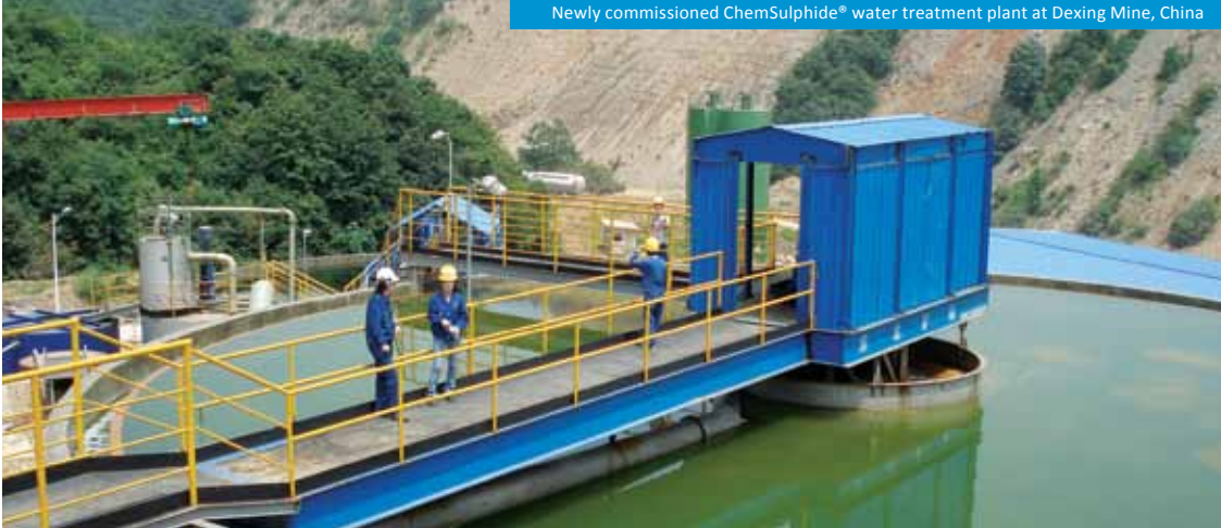
Newly commissioned ChemSulphide® water treatment plant at Yinshan Mine, China
