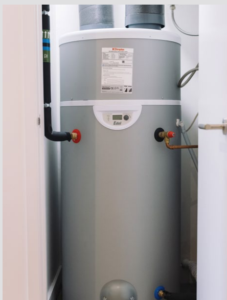
Air source water heater – Solstice Apartments, Milton Keynes
