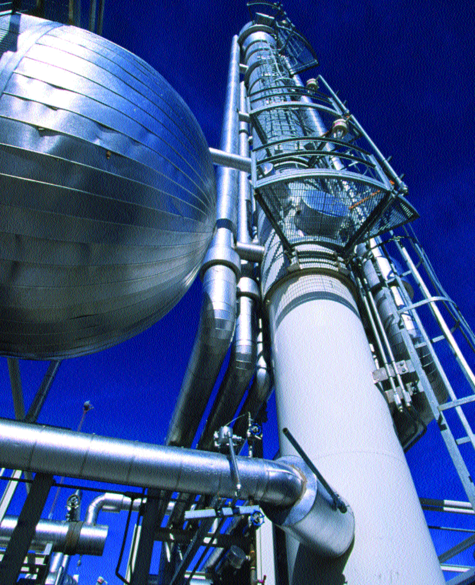
Devon's Bridgeport, Texas, gas plant processes the liquids-rich gas from our prolific Barnett Shale project. By owning and managing gas processing operations, Devon can enhance the economic returns of its development projects.
