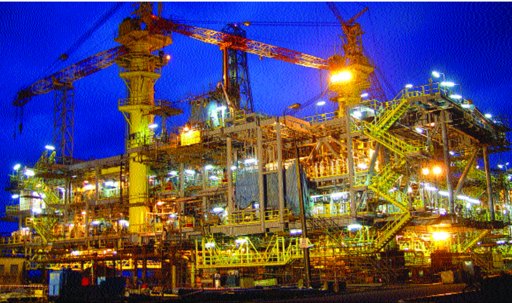
Offshore production facilities for Devon's Panyu project in the South China Sea are under construction in Singapore. Installation and first oil production are expected by year-end 2003.
