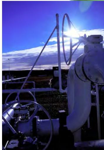
▲ THE HAVRE PIPELINE, managed by Devon, transports gas from our Bear Paw field in north central Montana. Devon owns interests in more than 13,000 miles of pipelines.
