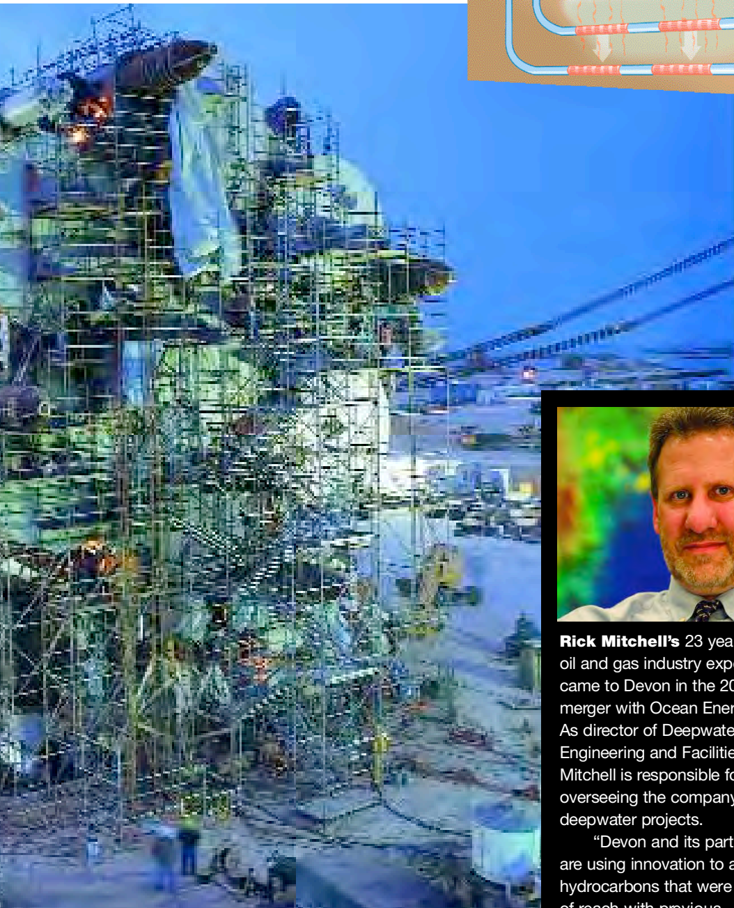
▲ CONSTRUCTION OF THE RED HAWK cell spar moves ahead toward a 2004 deployment date. The Red Hawk facility is designed to handle production of 120 million cubic feet of natural gas per day.
