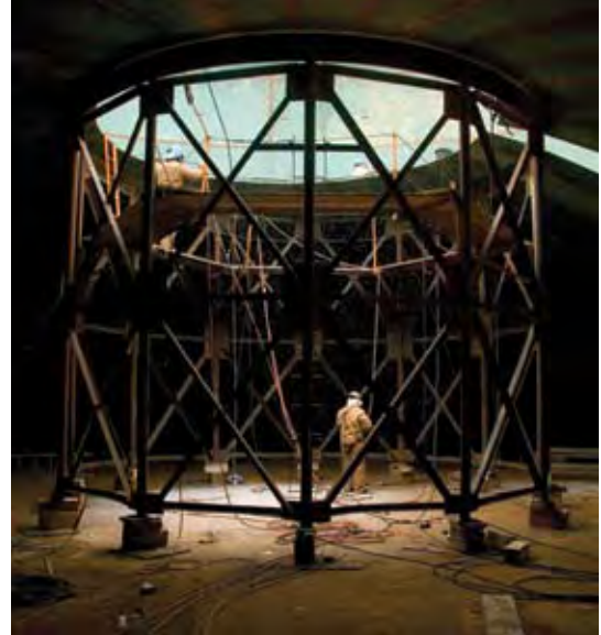
Welders construct facilities for Devon's Jackfish thermal oil sands project in eastern Alberta. Jackfish is expected to produce 35,000 barrels of oil per day.
