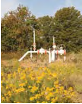
A Barnett Shale pipeline valve station is part of Devon's vast gas gathering system serving the north Texas area. Devon's cumulative operated Barnett Shale gas production surpassed one trillion cubic feet in 2005.
