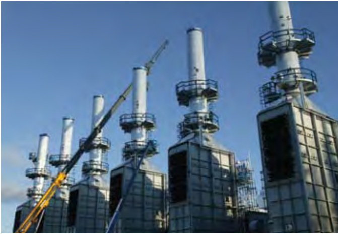
Construction nears completion at Devon's Jackfish thermal oil facility in Alberta, Canada. Commencement of steam injection and first production from Jackfish are planned for 2007.
