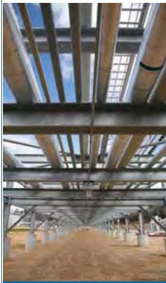
Tinsley EOR facility
