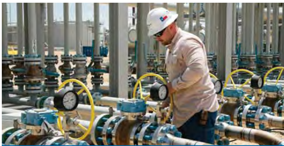
Operator at Hastings EOR facility
