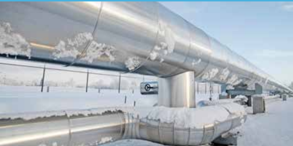
Steam from waste is delivered to our plants in pipelines.
