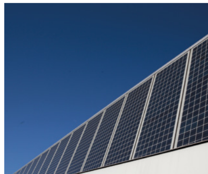
Riverbank House PV Cells
