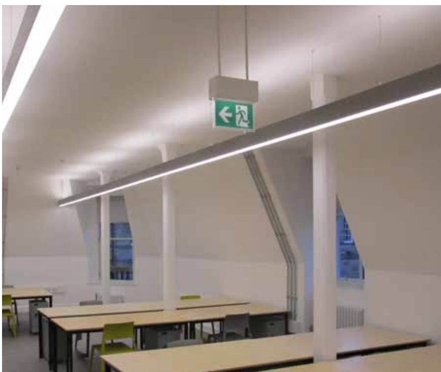
Specto XT installation at Chambers Square, Edinburgh
