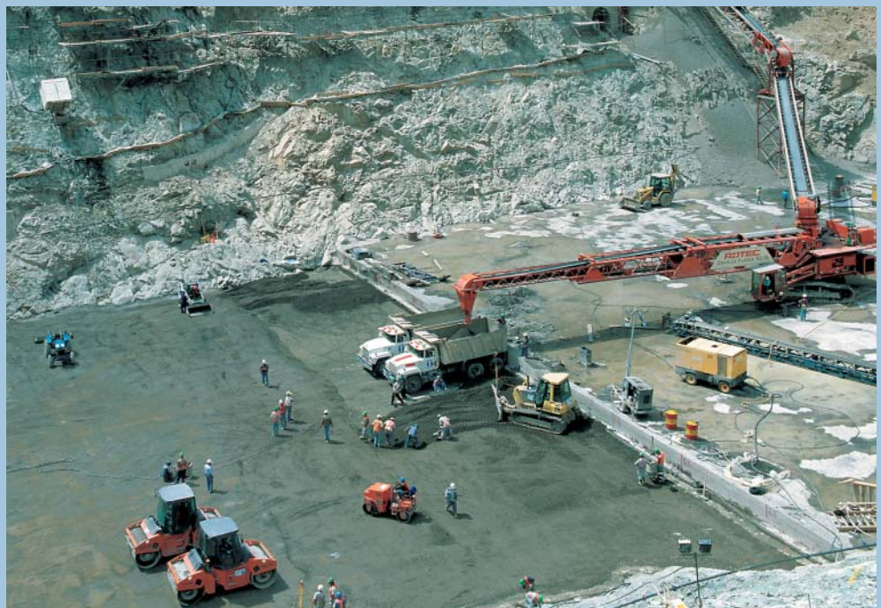
Ralco Power Plant Project, Chile
