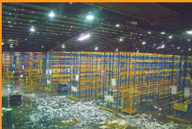
BEFORE : Hail damage at the Blacktown, NSW dry grocery warehouse in December 2007.
