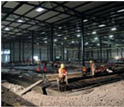
Our Hassloch, Germany, plant – which was devastated by fire on April 1, 2006 – is on schedule to resume production during the second quarter of 2007.
