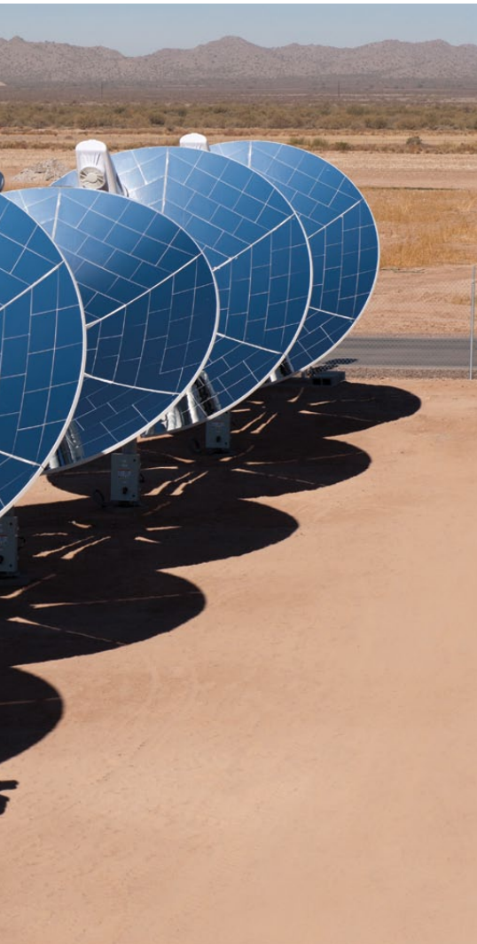
The solar power system at Frito-Lay's Casa Grande, Arizona plant is one way the facility hopes to operate almost entirely on renewable energy sources.
