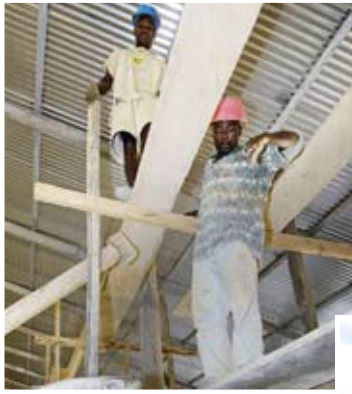
A community center is being built in one of the villages with Golden Star providing financial sponsorship.
