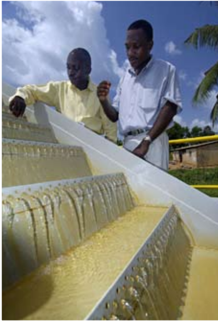
One of our nearby communities has too much iron in its water. Above we are commissioning a clarifying system to make the water potable.
