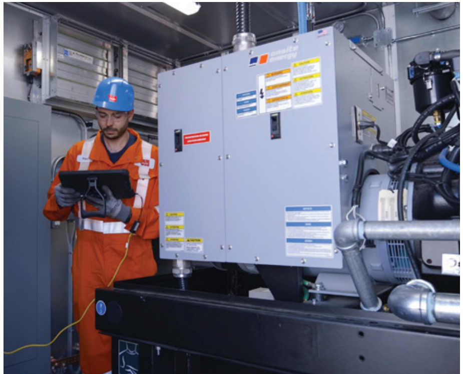
Power Generation Technician programming a controller to meet the customer's specifications, check warnings and shutdowns are working correctly.
