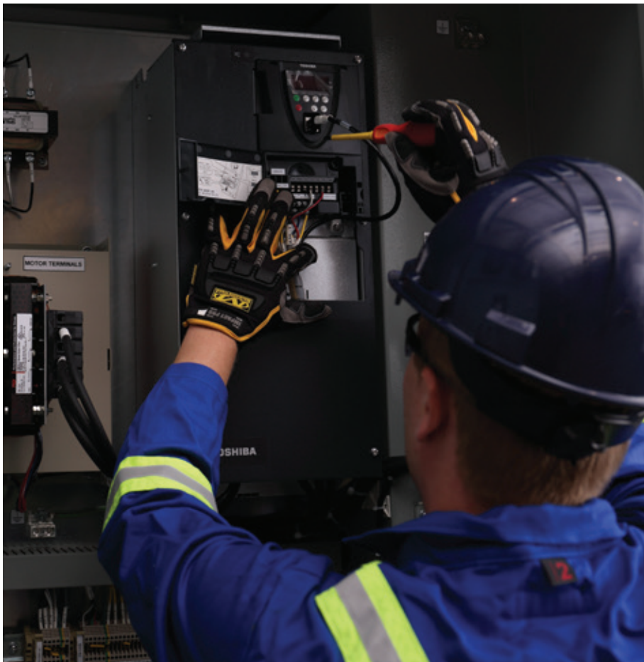
Senior electrician and controls technician at Tundra carrying out voltage and amperage quality checks on a variable frequency drive for a customer.
