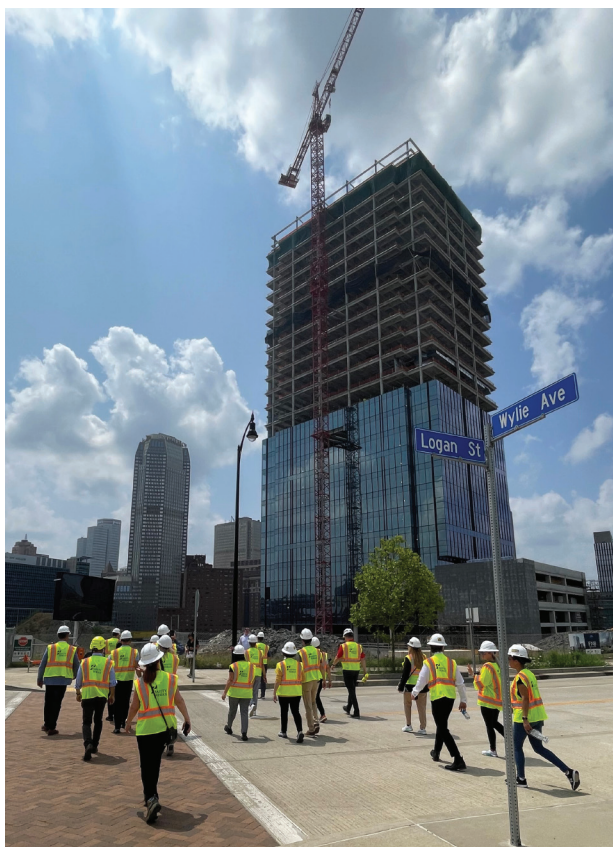
A group of FNB employees head to the FNB Financial Center site for a tour during construction.
