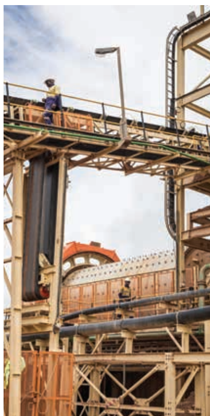
The ball mill at the Yanfolila process plant
