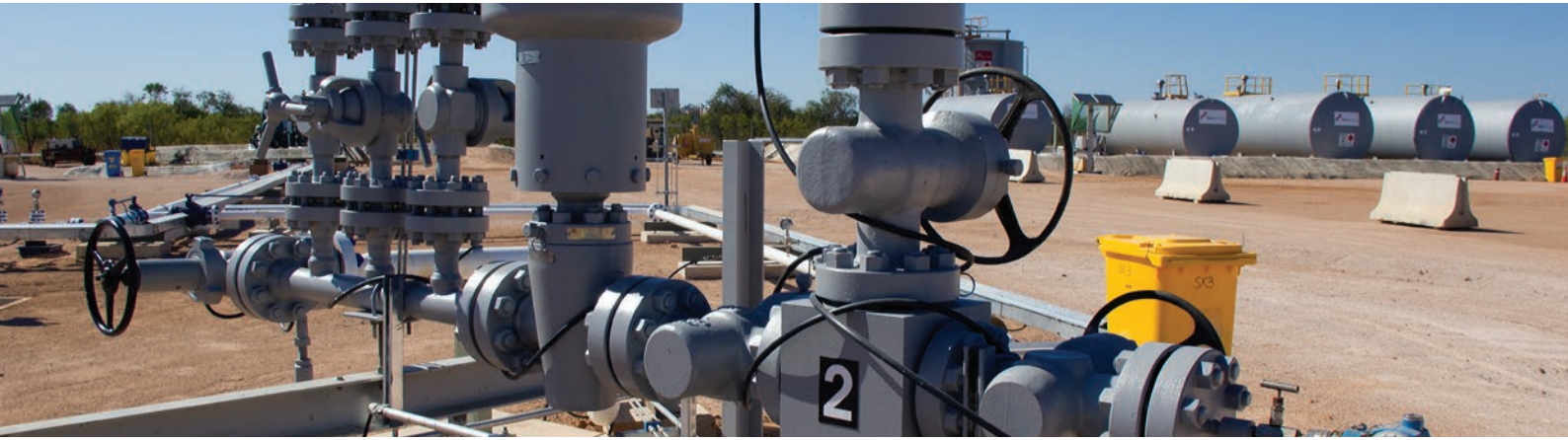
Ungani Production Facility
