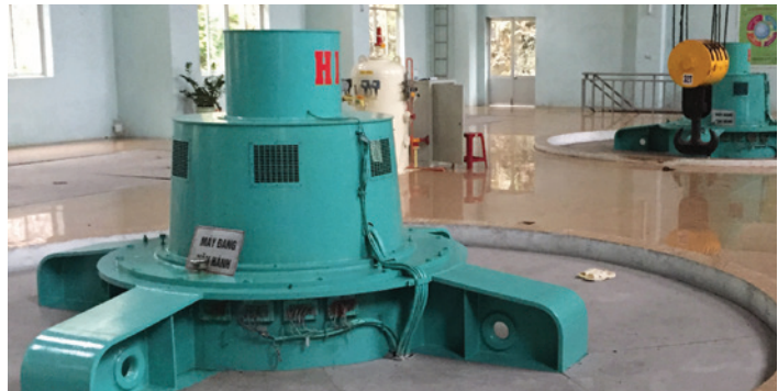
The power house supplies electricity for roughly 11,400 households in the region.
