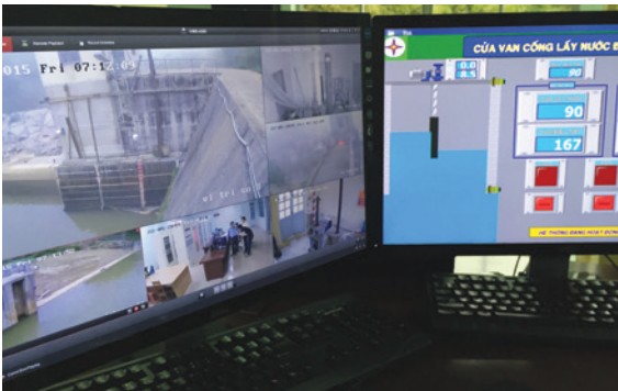
IT infrastructure in the central control room.
