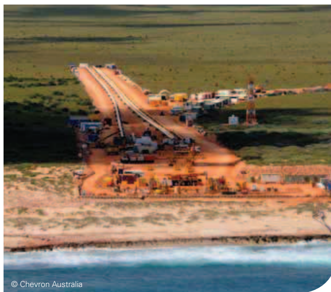
Pictured: Protecting one of the world's largest natural gas projects – Gorgon Project
