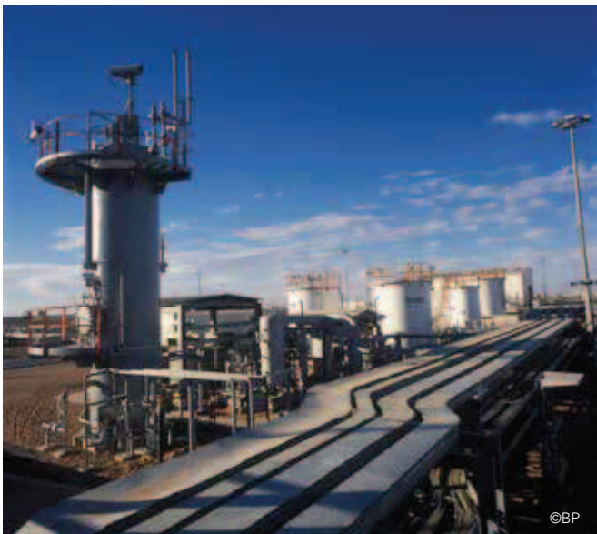
Pictured: Delivering complex and specialist surveillance solutions to serve requirements in hazardous areas
