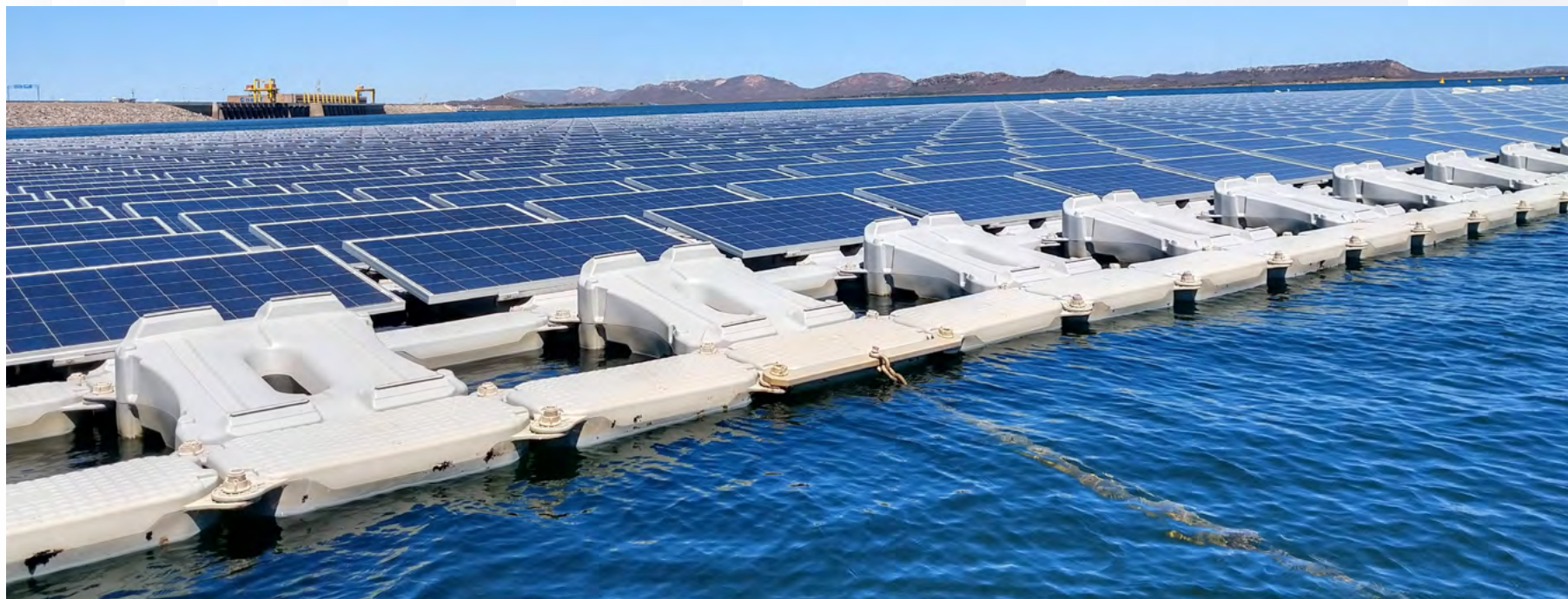
A Floating solar platform on an Eletrobras Chesf dam reservoir in Sobradinho (BA). Photo: Tatiana Leart.
