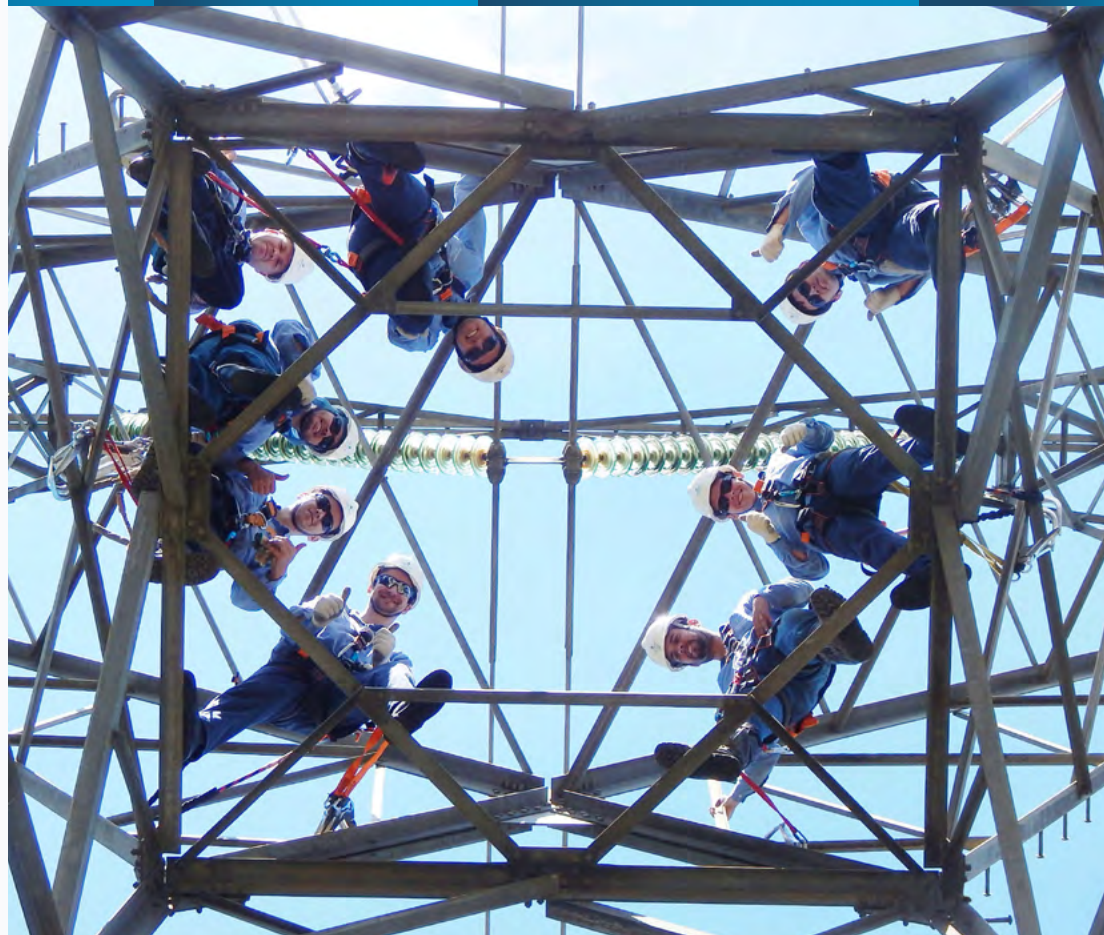
Eletrobras CGT Eletrosul linemen in training on a Blumenau-Curituba transmission line tower. Photo: Zezinho Mendes.
