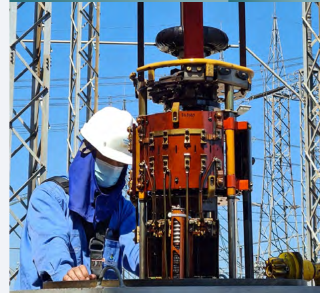
Servicing an Eletrobras CGT Eletrosul switch at the Curitiba Substation. Photo: Fernando Teodoro.
