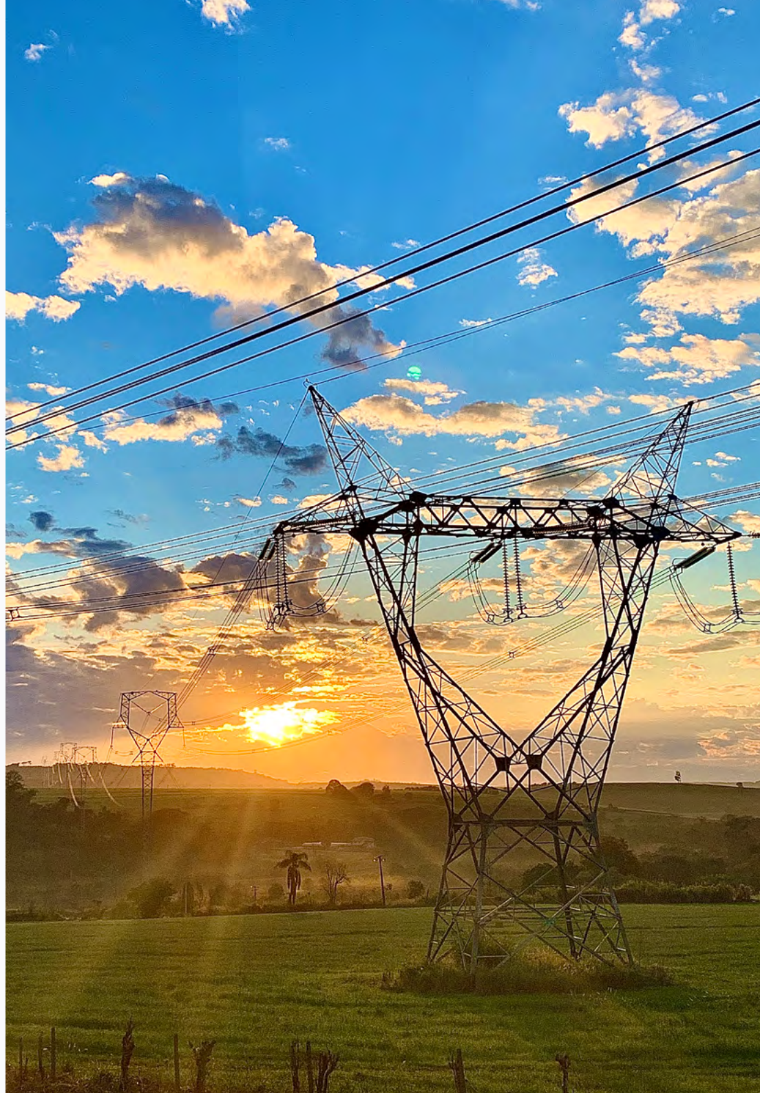
Eletrobras CGT Eletrosul's Londrina-Assis transmission line. Photo: Richard Souza.
