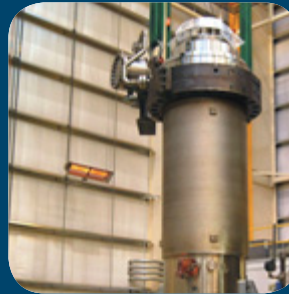
Electro-Mechanical Systems Reactor Coolant Pump
