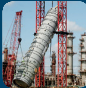
Oil & Gas Systems Fractionator
