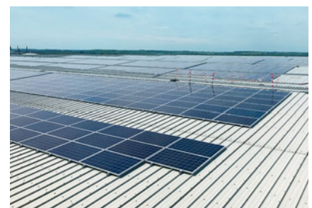
1,000 KW solar PV installation at our distribution centre in Newark let to Dixons Carphone.
