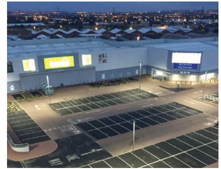
External car park lighting replacement programme at North Shields, completed in August 2016.
