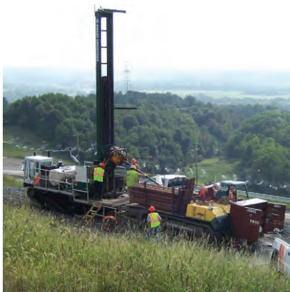
Boart Longyear is the #1 provider of drilling services to the US environmental industry.
