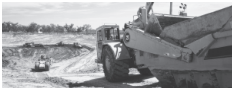
The primary crusher area at Cowal is excavated in preparation for construction. Production is expected in the first quarter of 2006.
