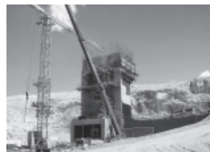
The primary crusher nears completion with an initial design capacity of 40,000 tons per day.
