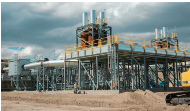
The Western 102 Power Plant, commissioned in early December 2005, is designed to lower energy costs at Goldstrike.
